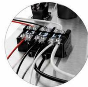
Terminal Block Detail
